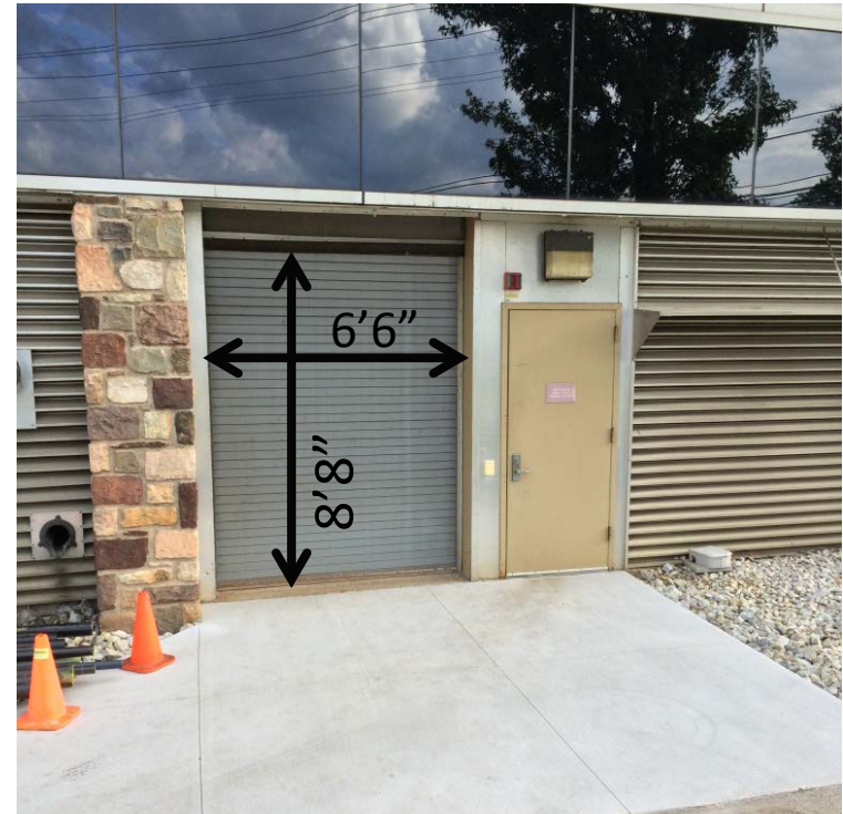
Access Doors to B38 Mechanical Room
