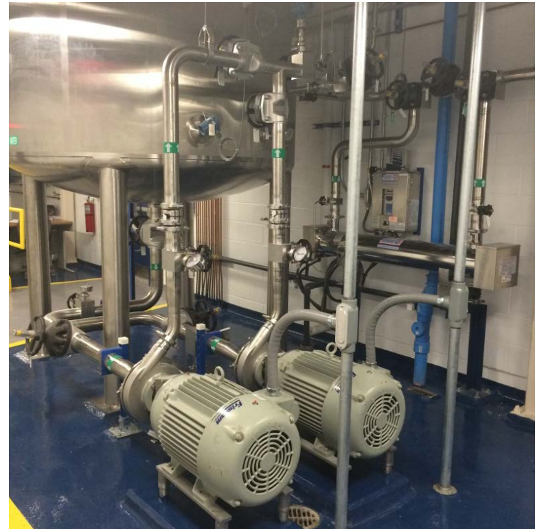
1 st Floor HPW Tanks & Pumps
