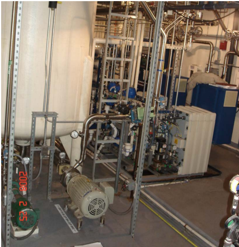
B38 Mechanical Room HPW System to Demo
