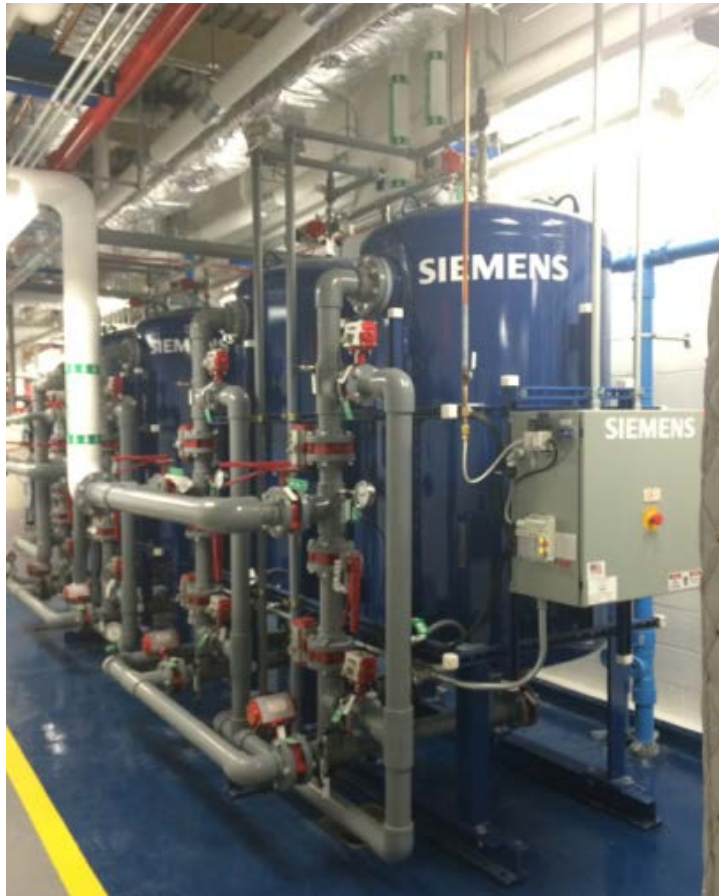
2 nd Floor Dual Softeners & Multi-Media Filters
