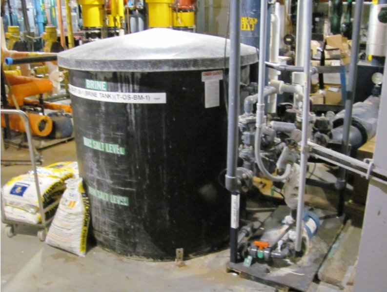
Softener Regeneration Brine Tank
