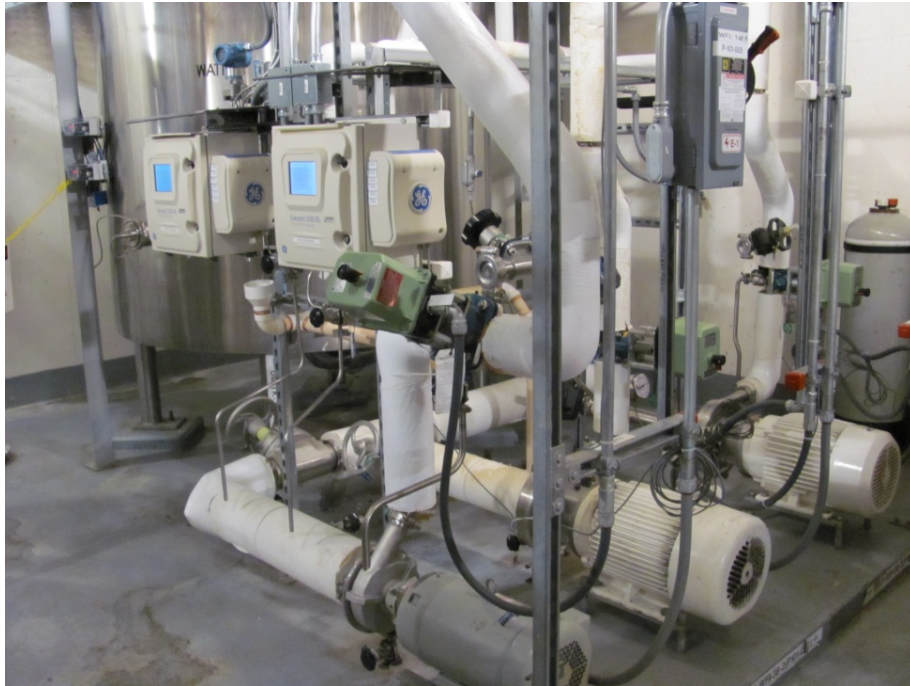
B38 Mechanical Room Existing WFI Pumps to Demo
