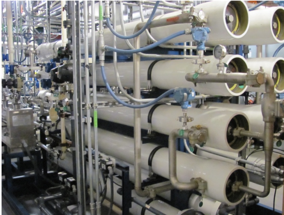
Reverse Osmosis Pre-Treatment System (Built c.1987)
