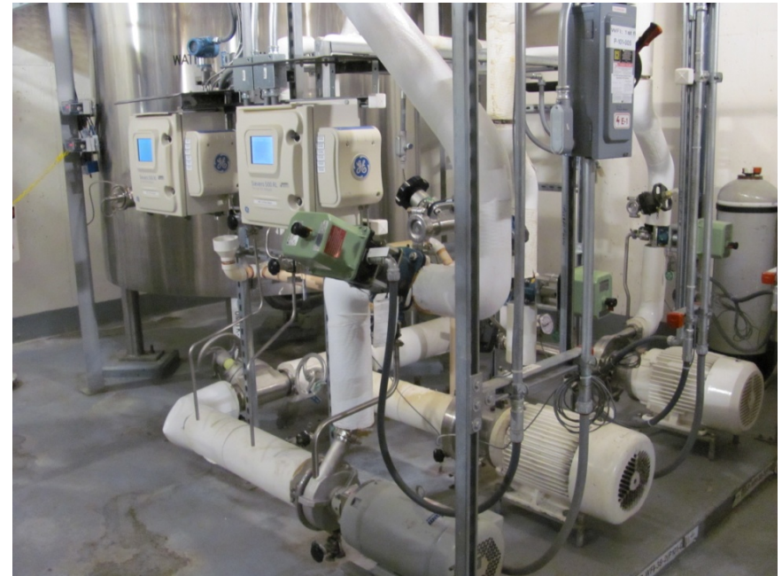
(3) WFI Distribution Pumps One pump on each floor (Spares in Warehouse)
