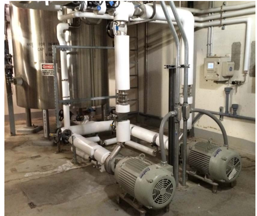
B38 Mechanical Room New WFI Pumps
