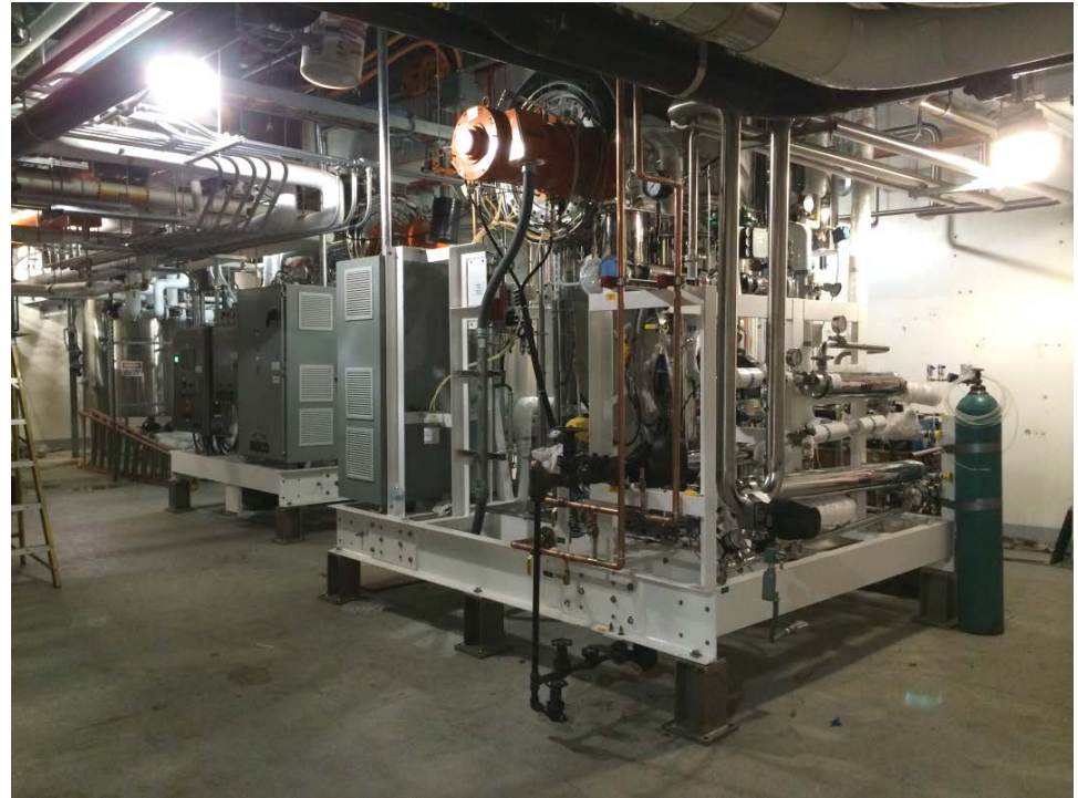
New WFI Stills in B38 Mechanical Room
