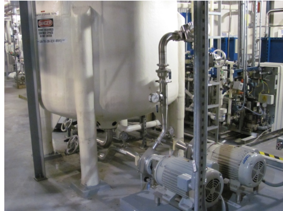
FRP High Purity Water Storage Tank 2000 Gallon (Built c.1987)
